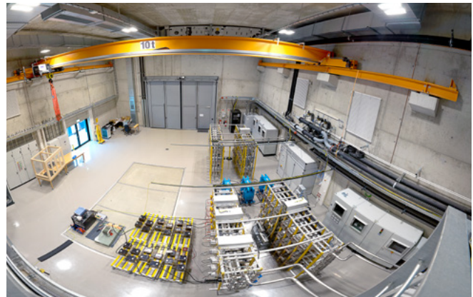
Medium voltage test lab with Modular Multilevel Converter (MMC) and high power supplies up to 30 kV and 3.2 MW © Anja Grabinger / Fraunhofer IISB
