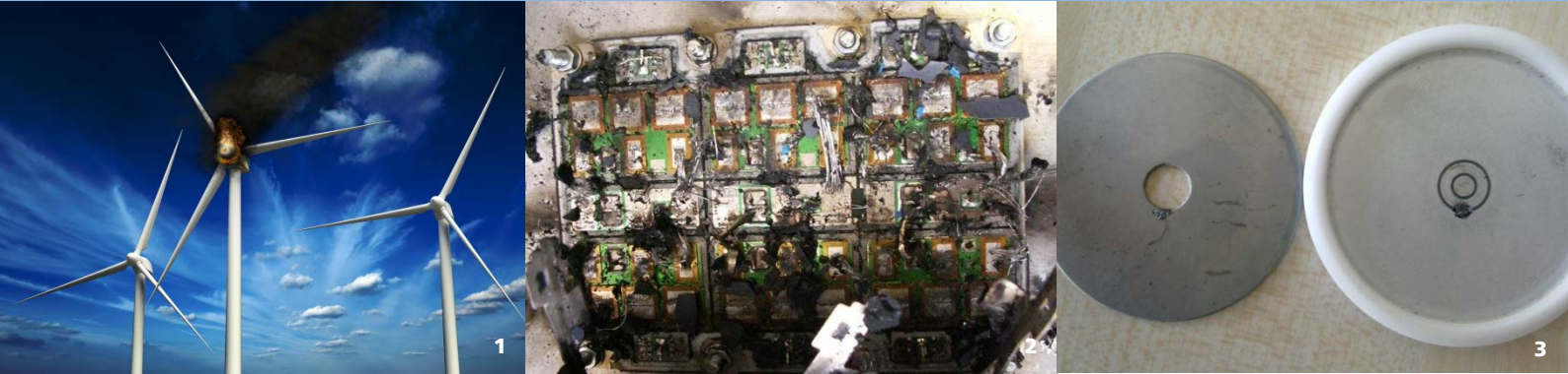
1 - 3 Examples of power electronic damages
